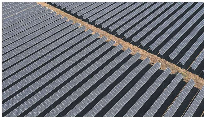
Saudi Arabia is building some of the world's biggest solar farms, along with giant arrays of batteries to store electricity. BLOOMBERG
