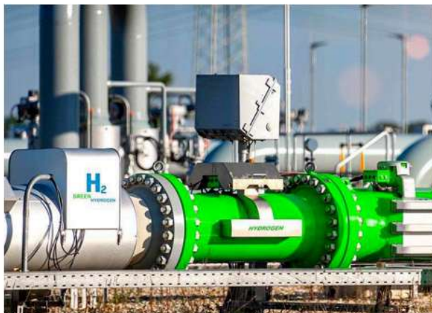
KEY INPUT. One of the major components in the cost of production is power, followed by operational expenditure
