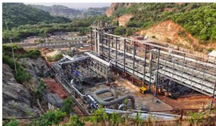
A view of ISPRL facility in Visakhapatnam
