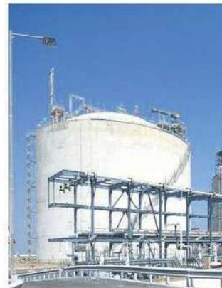
The Dhamra LNG terminal has regasification capacity of 5 mn metric tonne of LNG per year.
